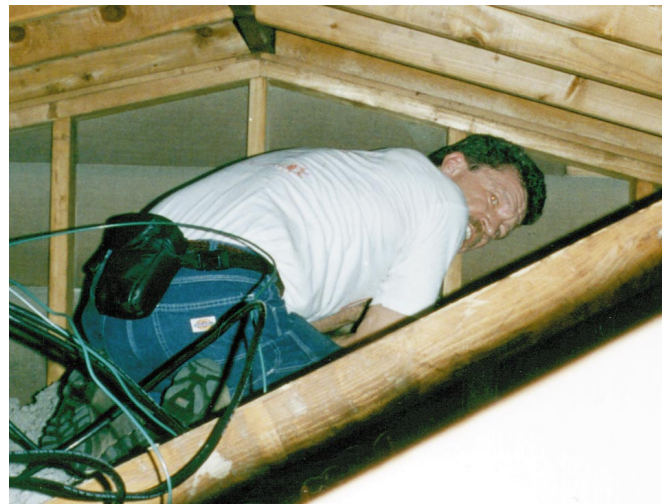
Above: Joe Flake of Go Solar Enterprises runs PV cables through Jane's attic. It is often small matters such as wiring that are critical and difficult. The hands-on training offered by SEI in their on-the-job courses gives their students experience in details such as safe and standard wiring practices. Classroom training is fine and necessary, but it must be backed-up with actual installation experience.
